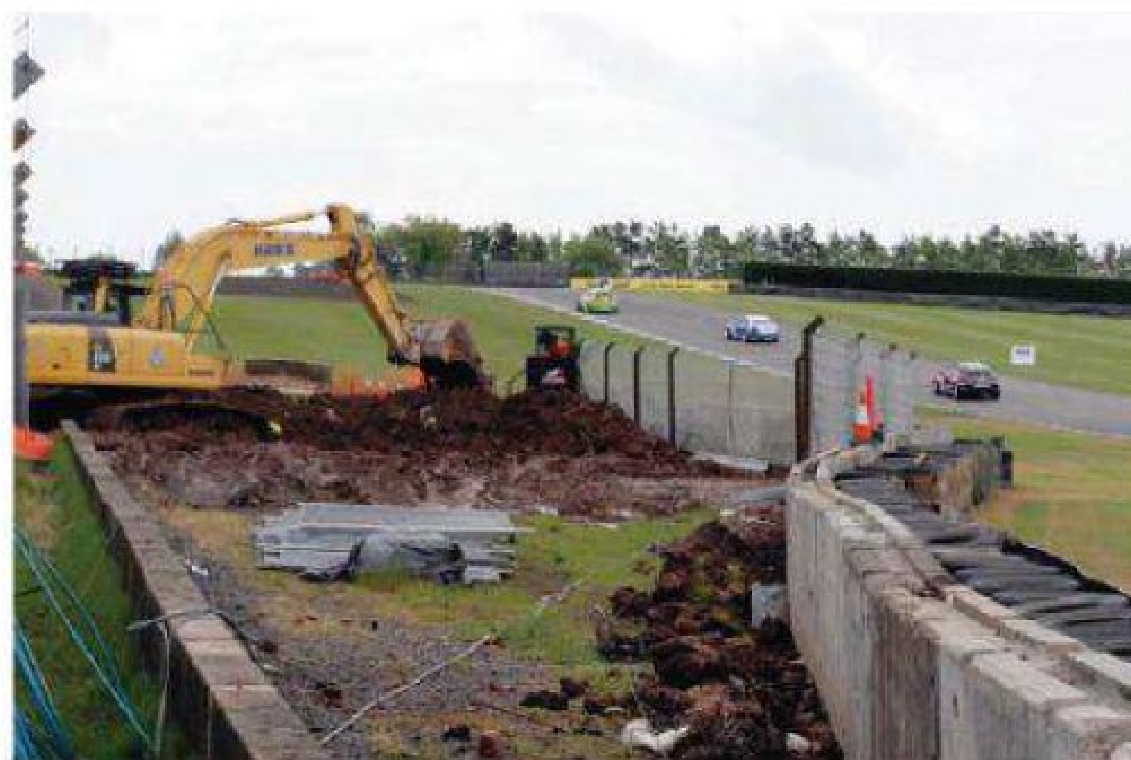
The first rule of building anything in England is get planning permission first. DVLL didn't, nor did it own the land it started unlawfully developing
