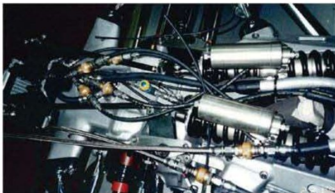
In this shot from the rear, the 'myriad hydraulic lines' are clearly visible
