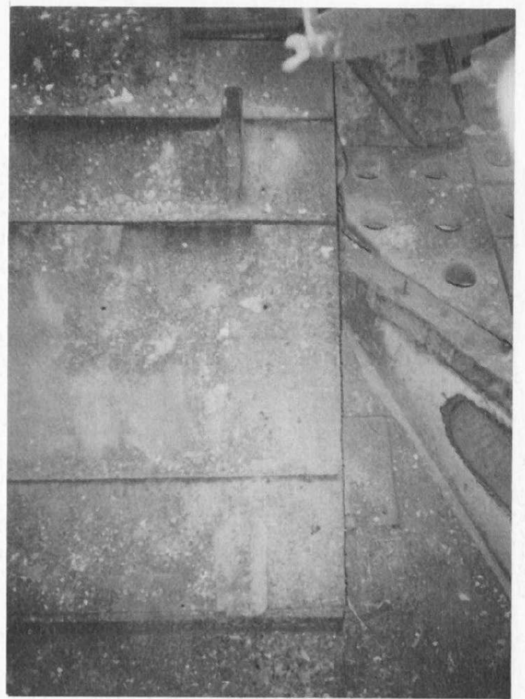
Although not the best angle, this photo illustrates a cross section of the rear angled plate that covered the electric motors for the drive sprockets. It is made up of four unequal pieces that overlap from top to bottom. This is looking towards the back of the vehicle.
