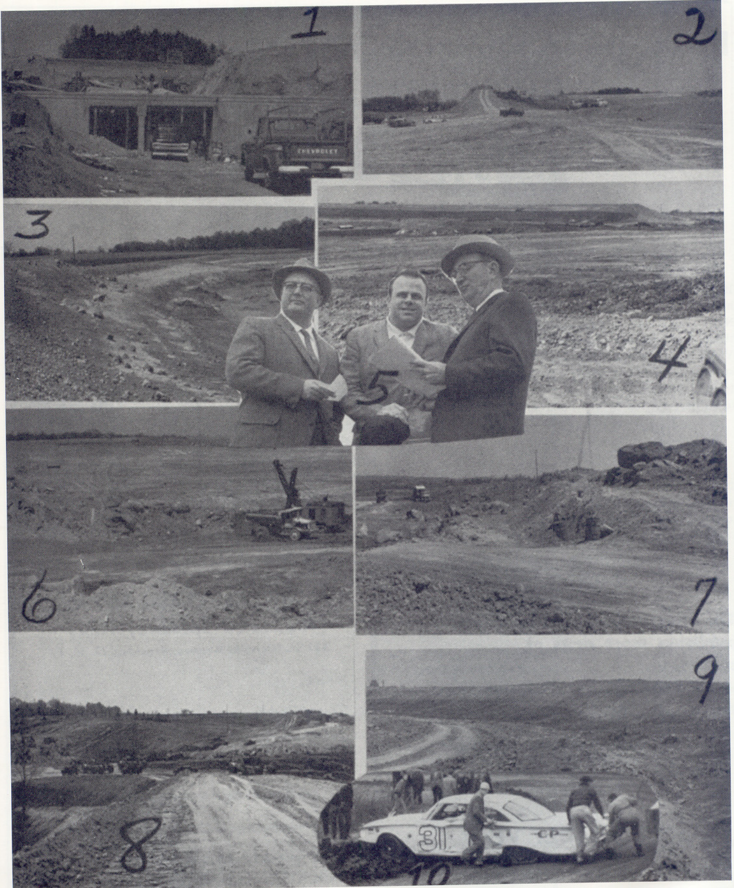
FULL-SPEED AHEAD — Here's the way Charlotte Motor Speedway looked the last week in April, 1960, as construction crews raced against the clock toward completion. 1. The sturdy tunnel beneath the fourth turn. 2. Looking at the site from the south end of the Ford Grandstand near the first turn. 3. Midway between the first and second turns. 4. Looking from the north end of the Chrysler Grandstand. 5. Bob Colvin (left), Darlington International Raceway president, and Bruton Smith (center), Charlotte Motor Speedway vice president, talk over racing plans with Champion Spark Plug Co. public relations director Dick McGeorge. 6. Rock removed from along the backstretch. 7. Looking at the second turn. 8. The backstretch and third turn take shape. 9. The fourth turn's 24-degree bank. 10. Crewmen work to get Johnny Beauchamp's car out back in a Charlotte Fairgrounds race.
