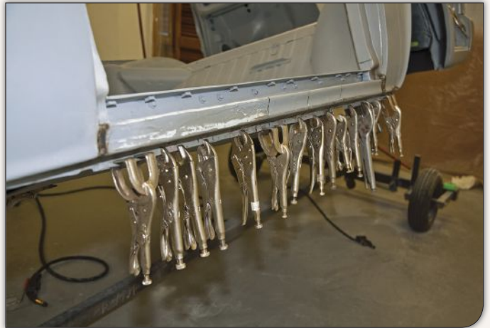
The Rampside's unique, mid-bed door gave the chassis an obvious weak point, the rocker panel essentially the only structure holding it together. More than a dozen locking pliers were required to keep the piece straight when welding it back together.
