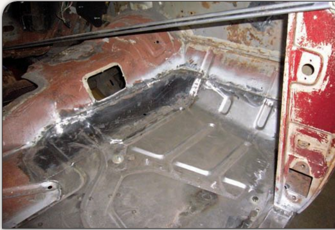
An aftermarket section of floorpan was obtained and carefully “dry-fit” into place for accuracy before the panel was first tacked into place via MIG welder. Sections at opposite ends were then completely welded to avoid warping due to excessive heat.
