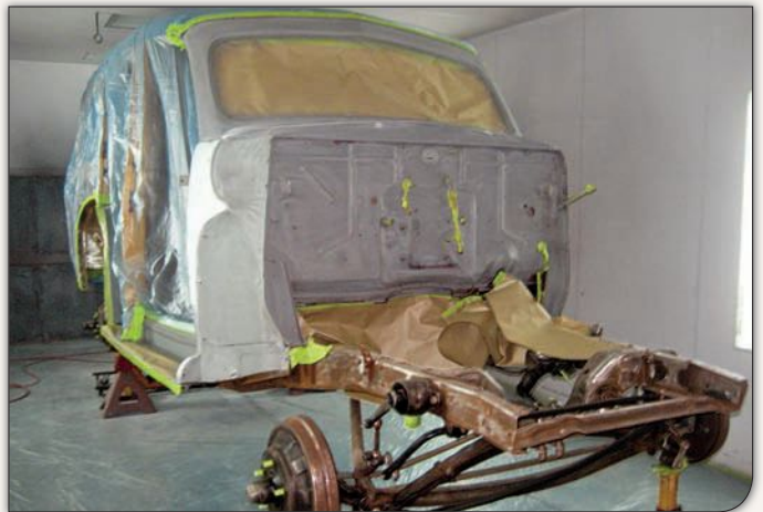
Even with the hood, doors and fenders removed, the restorers kept the rest of the body on the frame, even when restoring the frame. Using strip discs and localized spot sandblasting, the frame was thoroughly cleaned and prepped for refinishing.
