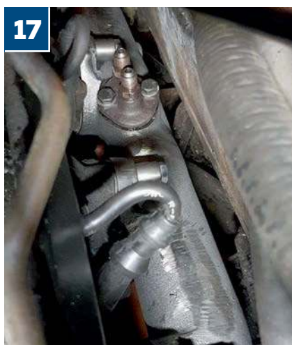
17 We're whizzing through the process here, but after agonising work removing the seized old equipment and working in the narrowest of spaces, the troublesome manifold was finally replaced
