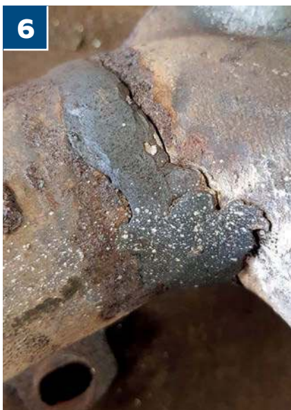
6 When the nearside manifold eventually came free, it was apparent the previously welded part had severely cracked
