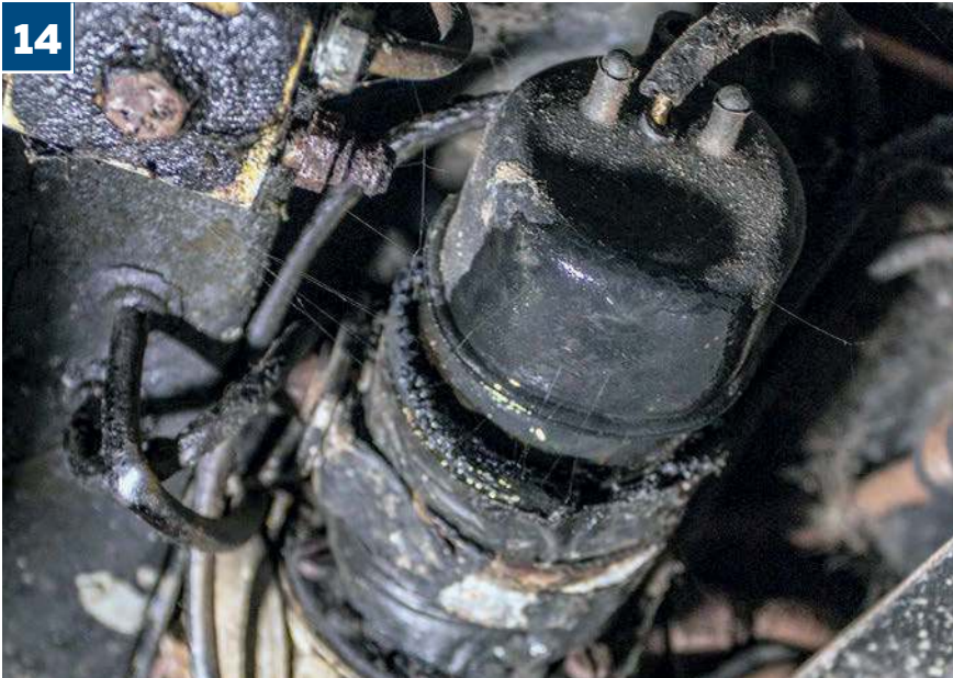
As this photograph demonstrates, the twin fuel pump assembly was seriously compromised; the rear pump had failed completely, the front pump was sending as much fuel to the floor as it was trying to feed the V8
